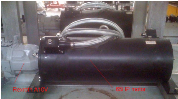
Figure.7. Hydraulic power unit
