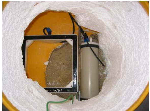
FIGURE 4: The topside WFS modem was mounted internal to the buoy hull, below the battery pack near the waterline deemed to be a safe location from fouling/corrosion.
