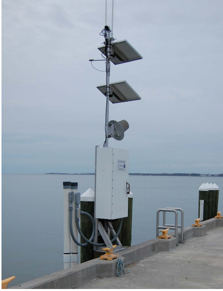
Fig. 1. Test water quality system on the VIMS Pier at Gloucester Point, Va., consisting of an electronics enclosure and mast with antennas and solar panels. The two PVC wells house the test instruments. The CBNERR reference sensor is deployed in the PVC well on the piling to the right of the test system.
