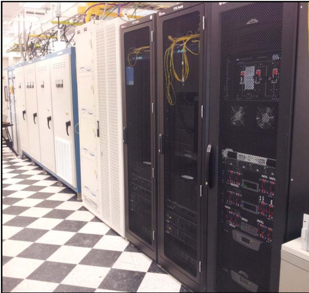
Fig. 8. RSN Shore Cabinet Line-up
