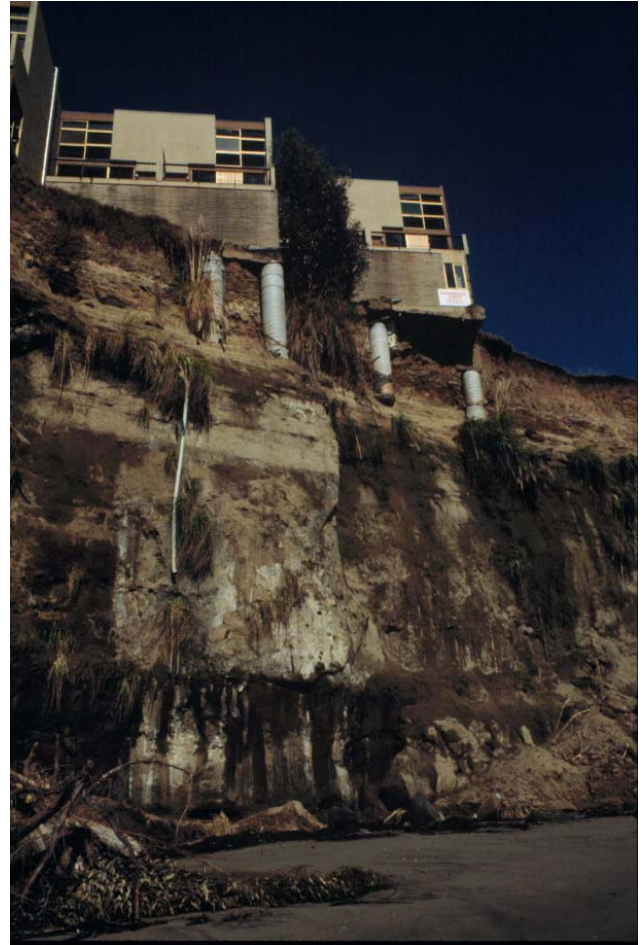
Fig. 12 Coastal cliff failure at Capitola during the Loma Prieta earthquake led to demolition of these apartments.
