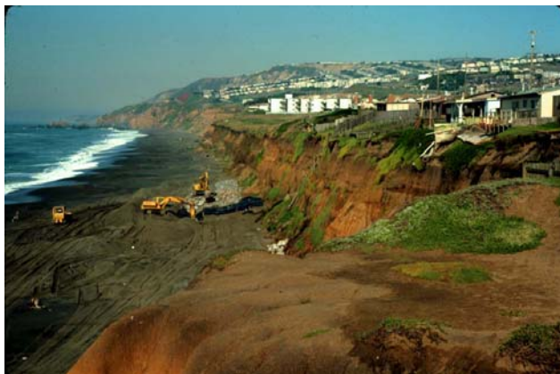
Fig. 13 Bluff failure in Pacifica during the 1982-83 El Niño winter.
