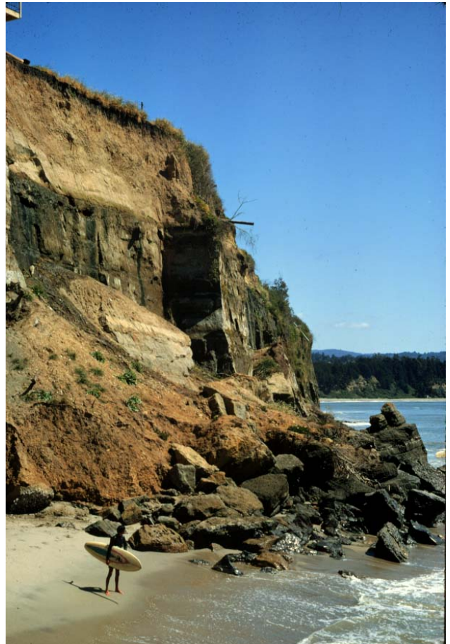
Fig 9. Large-scale cliff failure along joint sets in Northern Monterey Bay.
