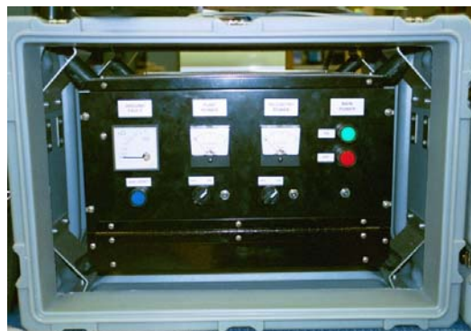
Fig. 8: Topside Power & GFI Console
