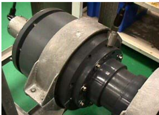
Fig. 4: Main pump & flowmeter assembly
