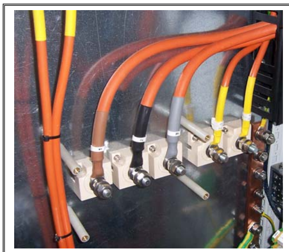
Figure 2 - High Voltage Umbilical Termination Unit
