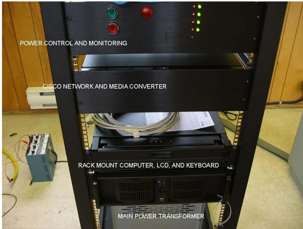
Shore Station Equipment Rack
