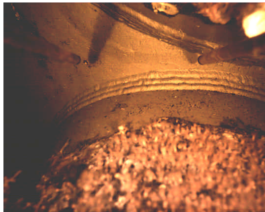
A weld inspection shows metal pitting
