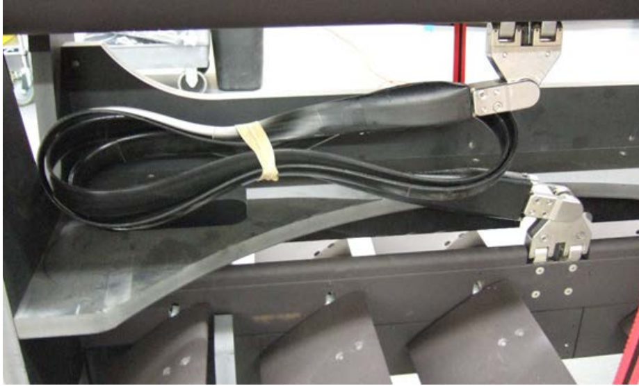
Figure 10.9. Banded Umbilical Resting on Launch Saddle Frame
