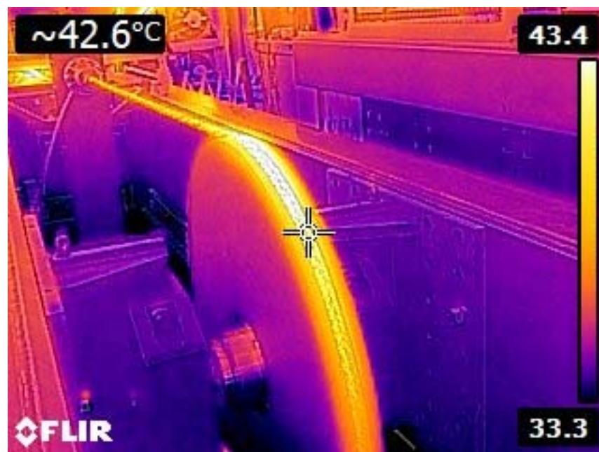
Figure 9.8: Example thermal image taken during checking of the cable external temperature.
