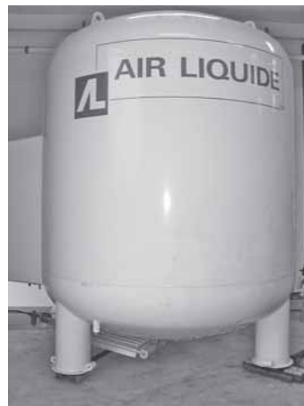
Nitrogen tank for the cooling system
