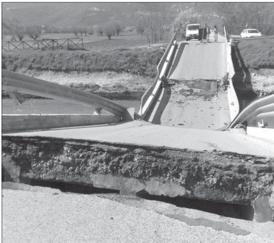
The vulnerability of steel and concrete bridges, such as this bridge over the Aterno River, was underscored by the earthquake in Italy on April 6, 2009.
