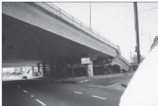
During the January 17, 1994, Northridge earthquake near Los Angeles, Calif., a section of I-10 collapsed.
