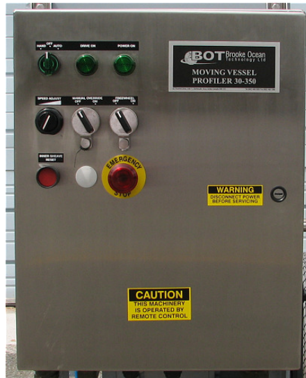
Main Control Box
