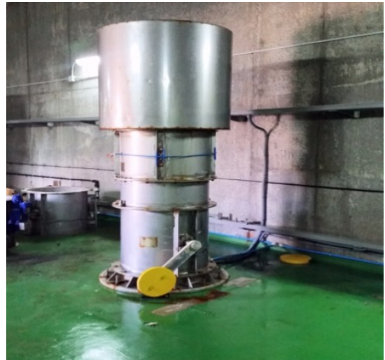
Fig.1. Turbo-generator modules in Mutriku wave plant
