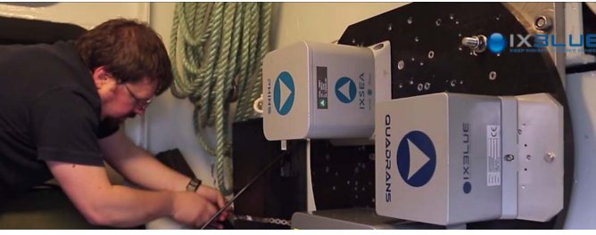
Fig. 3. Inertial systems mounted on the wall
