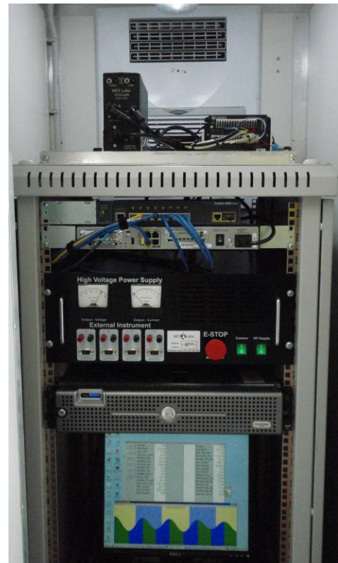
Figure 6. Image of the computers, communications and power supply devices installed in the 19" rack in the air-conditioned cabinet.
