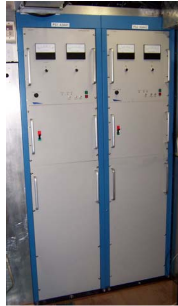
Figure 8. DTI COTS 200 kW, 20 kV power supplies.
