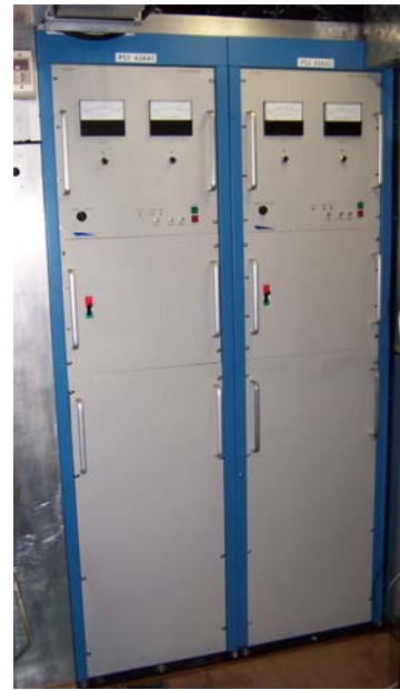
Figure 8. DTI COTS 200 kW, 20 kV power supplies.
