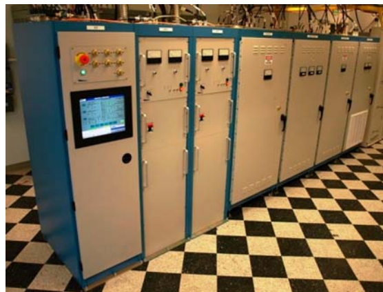
Figure 2. Installed Shore Power Feed Equipment.
