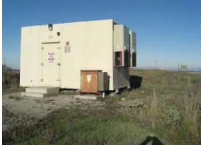
MARS high voltage cable termination hut
