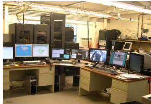
The MARS control room
