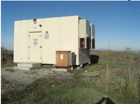
MARS high voltage cable termination hut
