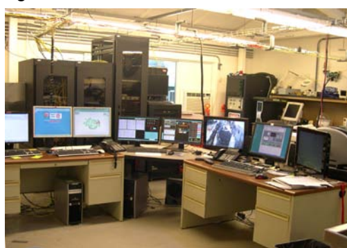
The MARS control room
