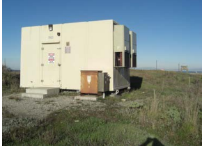
MARS high voltage cable termination hut
