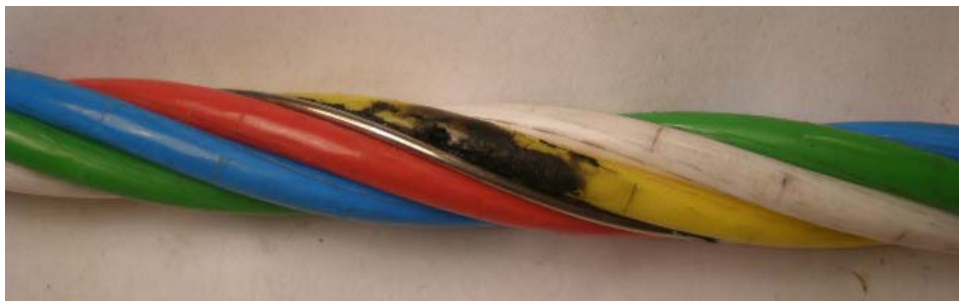
Failure #3 in Yellow Cable
